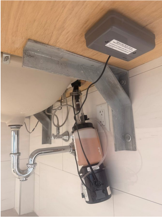
Galvanized steel angle bracket, wall-fastened, supporting the plywood underside - the bracing method shown on A-15. Confirm bracket size/spacing on site; not dimensioned on the drawing.
