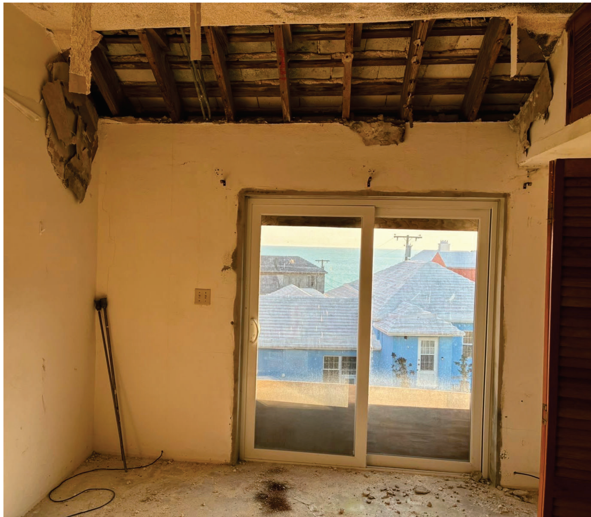
I.5 A0.02 INTERNAL IMAGE EX. CEILING DAMAGE
